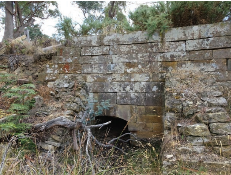
Downstream side of a culvert on the hill behind Woodsden. The two early buttresses indicate that the quality of engineering was not high (Malcolm Ward)
